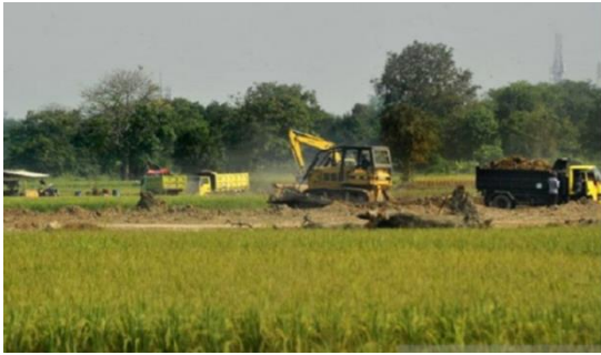
Workers with heavy equipment bury rice fields to be converted into housing areas. Dock. ANTARA/Asep Fathulrahman
