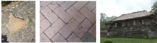
Figure 6. Damage at Taman Ayun Temple Source : Suryada, 2026
