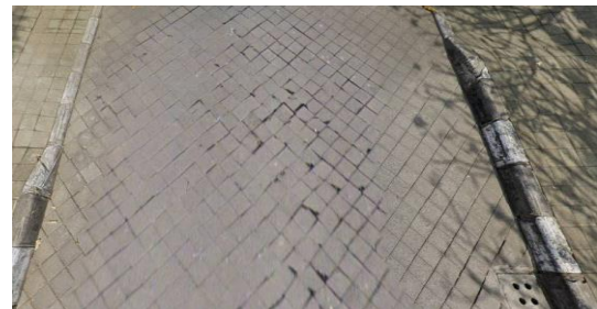
Figure 8. Damaged paving blocks on Ayodya Streets Source : Google Earth 2026
